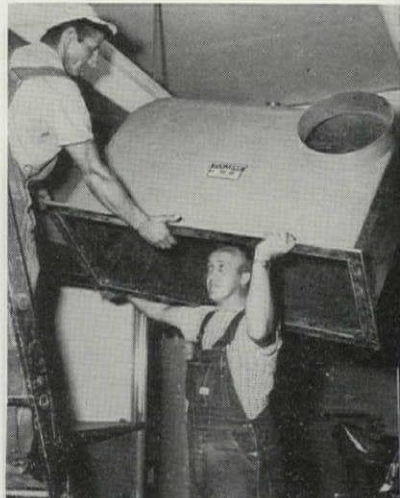
Figure 7. Workmen fit plenum chamber, first stage of duct system made of reinforced polyesters.
