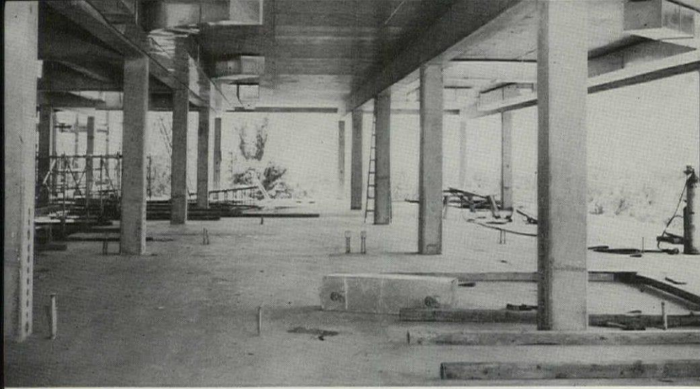
Figure 5. An unforeseen financial gain developed through the use of plastic coated plywood as form material. Greatly expanded re-use, plus reduced cement finishing after forms were removed, offset higher cost of form material. Smooth surface ceilings, as above, requiring no additional finishing are typical.
