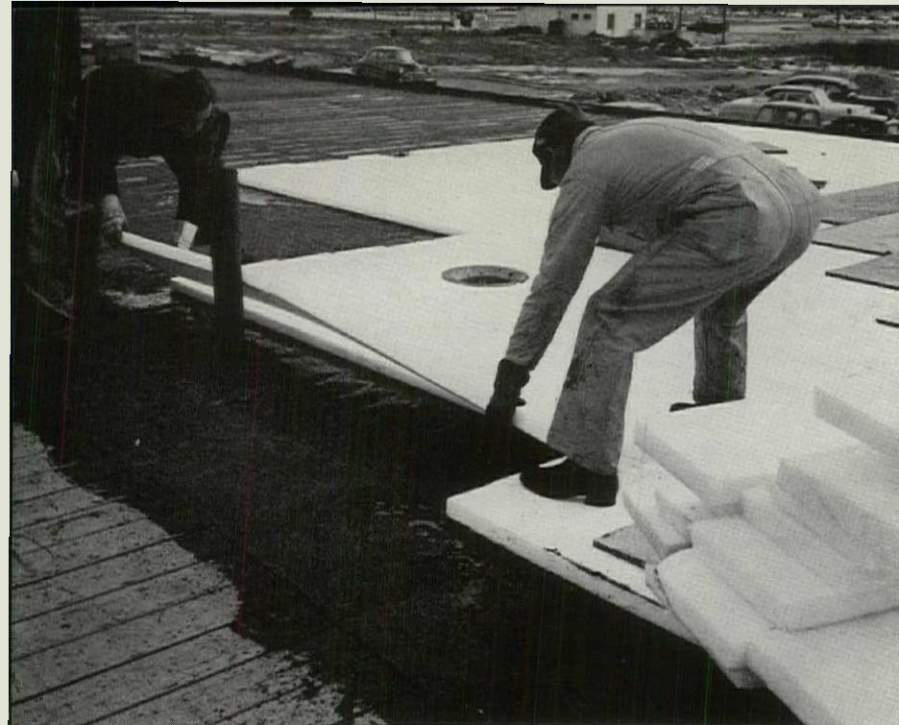
WORKMEN LAY POLYSTYRENE FOAM BOARD IN \frac{1}{2} " ADHESIVE OVER FELT OR FIBERBOARD AS A PROTECTIVE LAYER.
