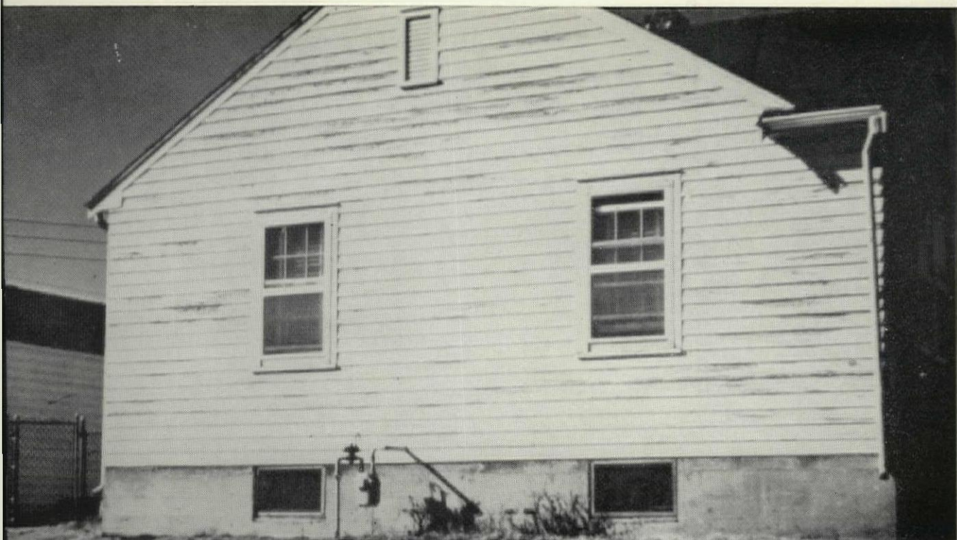
Blistering and peeling paint is one of the most common types of damage caused by the collection of excessive vapor in the side walls.
