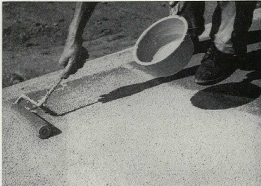
HYPALON SOLUTION WAS FIELD APPLIED WITH STANDARD PAINT ROLLERS TO THE NEOPRENE-COATED ROOF USED IN THE NAHB RESEARCH HOUSE.
