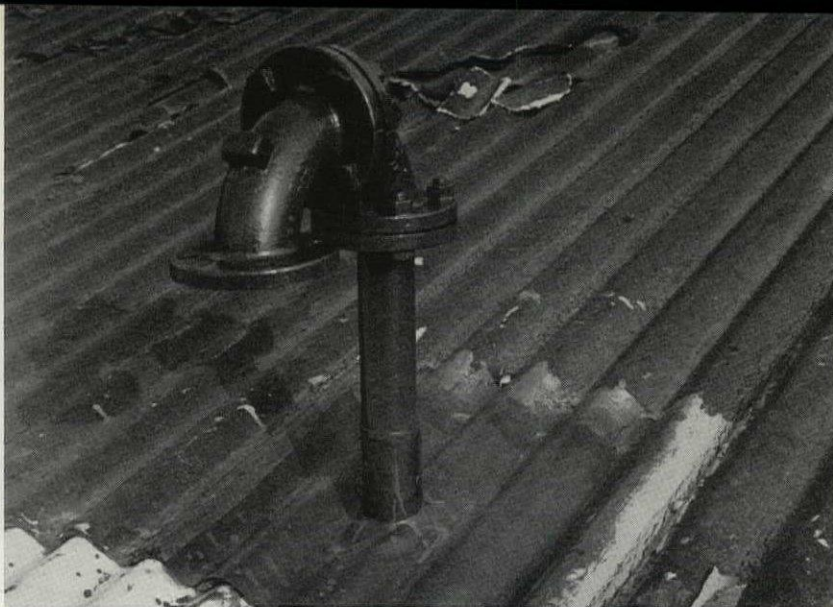
FIGURE 3. VENT STACK FLASHED TO CORRUGATED ROOF WITH PLASTIC FLASHING
