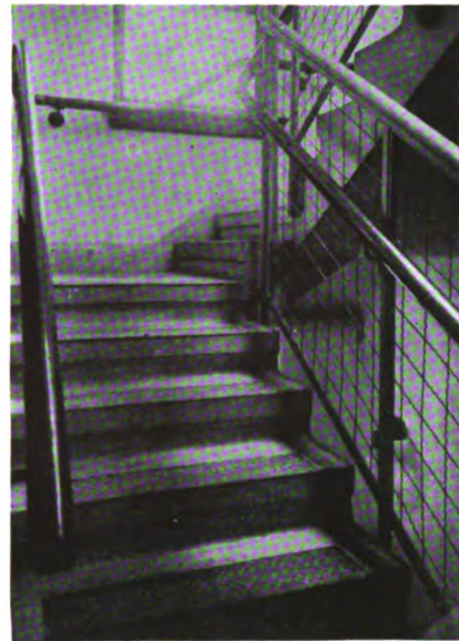
Approved Construction—"FERALUN" in Concrete Steps
