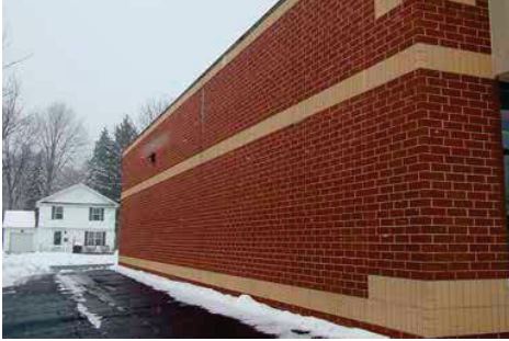
A building with cavity insulation, but no C.I.
