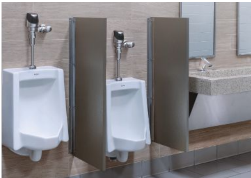
Corning Painted Post school district installed battery-operated sensor flushometers and turbine-powered faucets for a high-quality, easily serviceable and touchless environment. Photo courtesy of Sloan Valve Company
