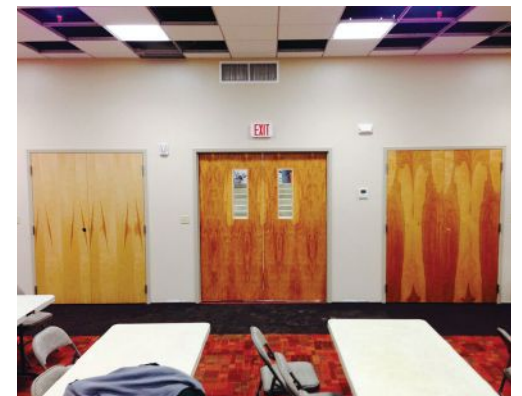
Problem of mismatched veneer doors in commercial application.
