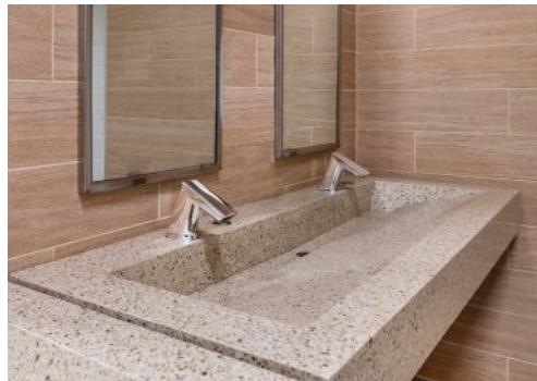
Corning Painted Post school district installed turbine-powered sensor faucets for a unique look, in addition to hygienic and water-conserving benefits. Photo courtesy of Sloan Valve Company
