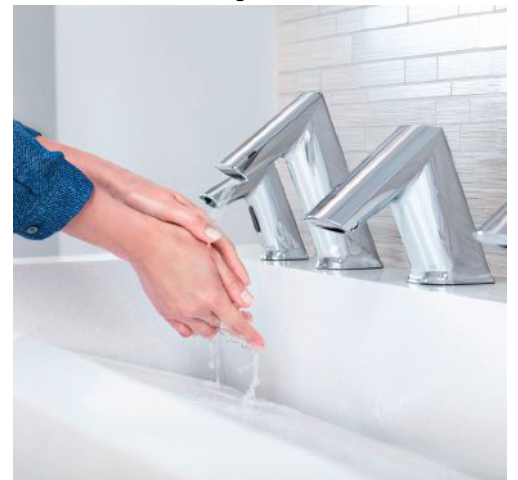
Sinks with integrated faucets, soap dispensers and hand dryers are appearing in classrooms, cafeterias, public areas and restrooms. Photo courtesy of Sloan Valve Company
