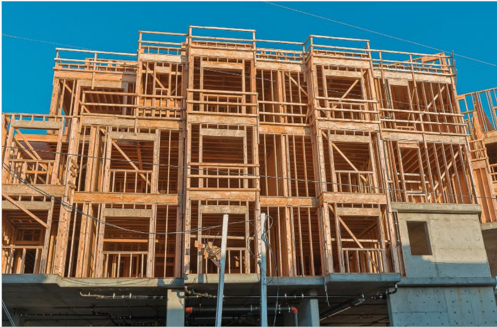
Typical light frame roof and floor systems consist of repetitive framing members such as rafters or trusses with wood structural panel decking. Photo courtesy of Think Wood
