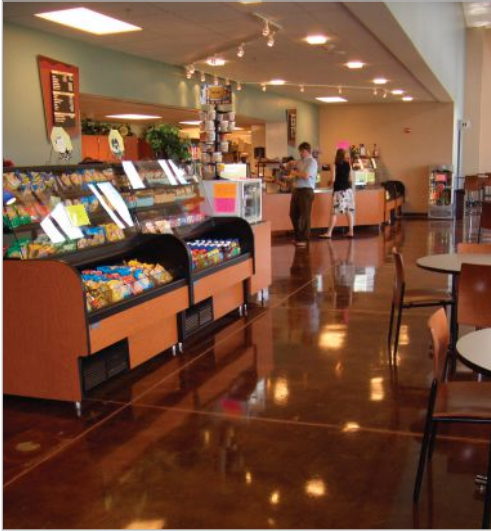
Interior joints on horizontal surfaces that see traffic such as this decorative stained concrete floor can be sealed to make cleaning easier.
