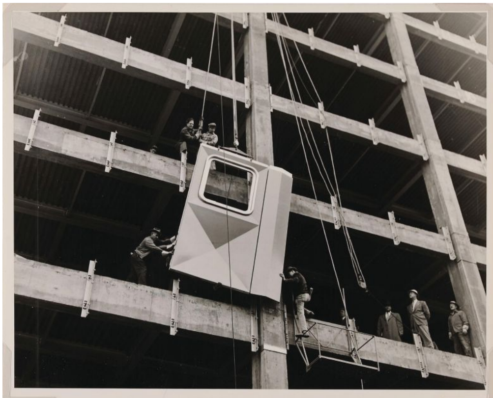
ABOVE: Workmen install the first aluminum panel on the Alcoa Building (now the Regional Enterprise Tower) in Pittsburgh, 1951. | BELOW: Mark Pasnik says that projects like the Alcoa Building are an important part of Pittsburgh's legacy and preservation's alignment with sustainability.
