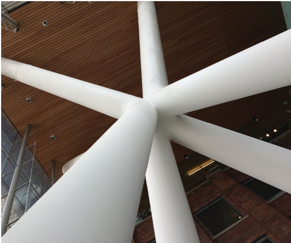
Architecturally exposed structural steel used on buildings of all types can now also be true design statements due to the availability of cast steel connectors in the US and Canada. Photo courtesy of CAST CONNEX
