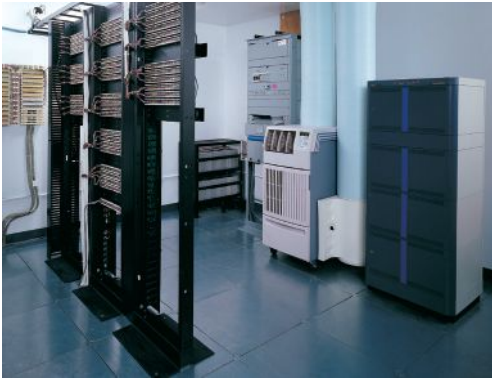
Spot coolers provide a convenient and cost-effective way to cool server rooms where equipment must be kept at a certain temperature. Photo Credit: MovinCool
