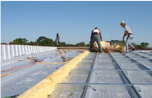
The cavity between the old and new roofs can be used to add insulation. Photo Credit: Roof Hugger
