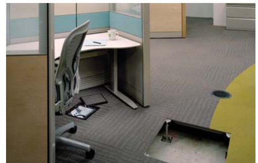
The underfloor air distribution system used in this BP Amoco building in Houston—dubbed BP WOW (Working Our Way) not only helped earn the building a LEED certification, but also makes future renovations easier and more cost-effective.
