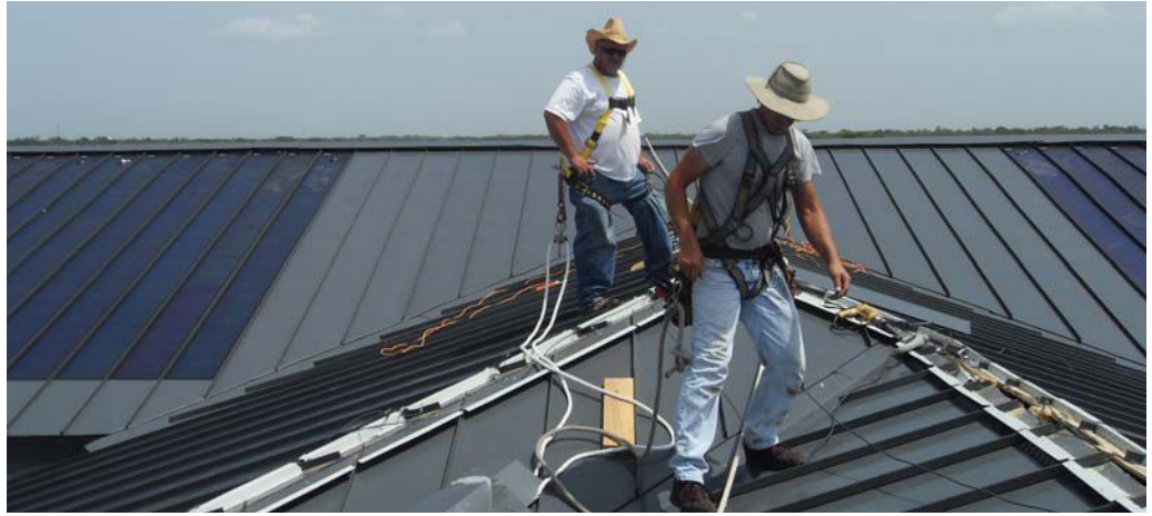
The decades-long service life of standing seam metal roofs makes them ideal for rooftop solar installations. Whether with crystalline photovoltaic arrays or thin film laminates (as pictured here), metal allows PV systems to be installed without creating roof penetrations. Photo Credit: Drexel Metals
