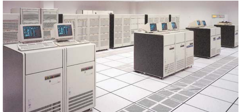
A data center from the 1960s to 1970s
