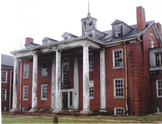
Emery Hall, by architect Frank Packard, was built in 1913 for Ohio's Wilberforce University, the oldest private black university in the nation. Currently owned by Central State University, the building was added to the National Register of Historic Places in 2005.
