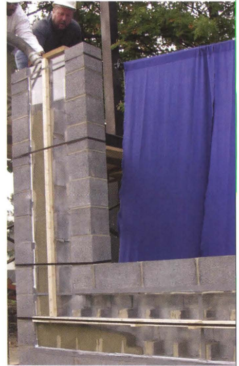
Self-consolidating grout (SCG) moves freely in tight spaces, as seen through the clear plastic face on this demonstration panel.
