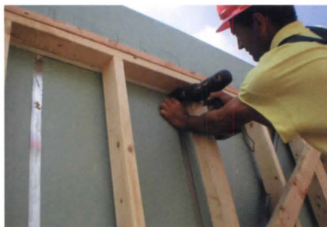
A construction worker attaches an aluminum clip that connects the area separation wall to the adjacent wood frame structure.
