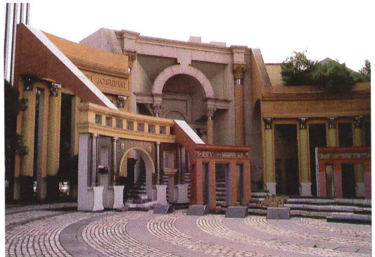
Charles W. Moore's Piazza d'Italia is in a state of disrepair.
