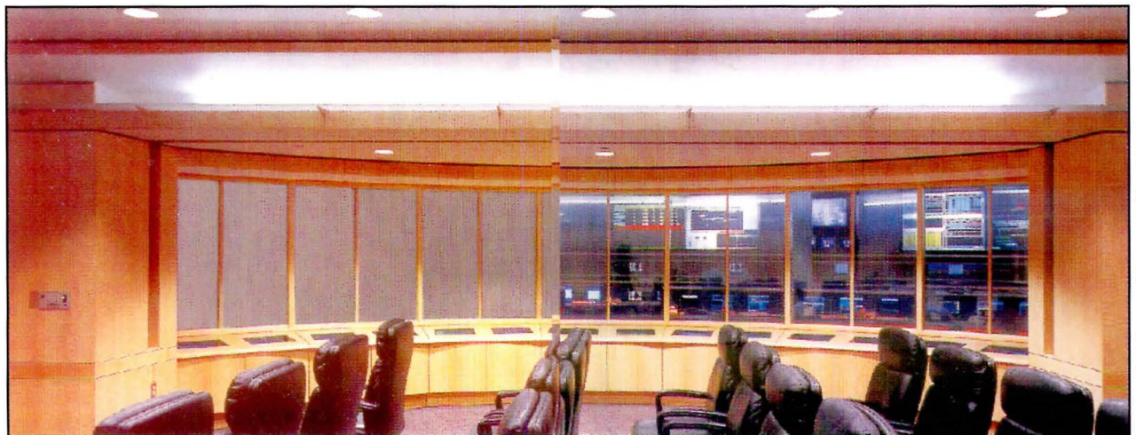
IBM Command Center - Boulder, Colorado
