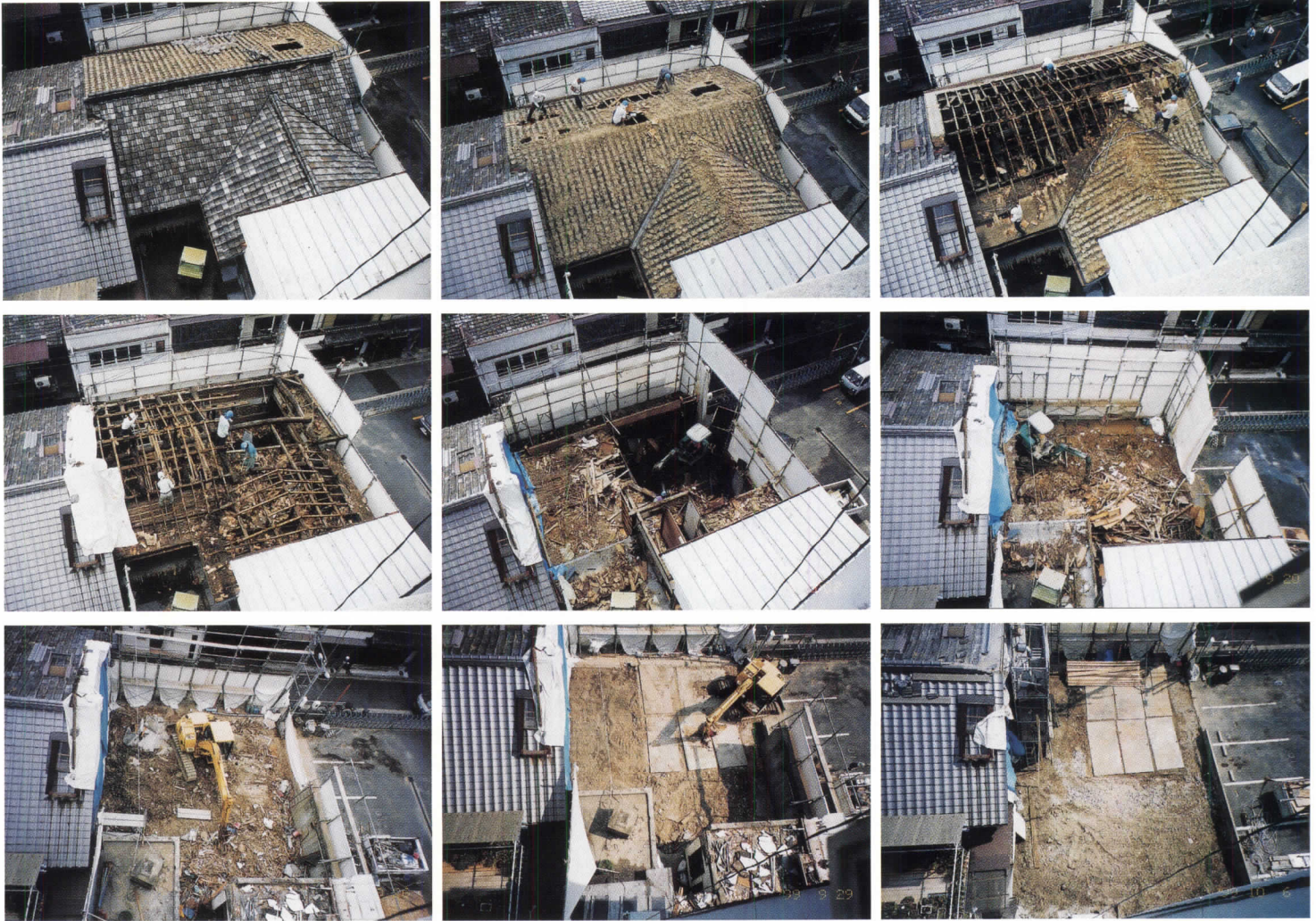
Workers begin demolition of a 70-year-old machiya by stripping away its tile roof and the underlying layer of clay. Chainsaws are used to sever beams and rafters. A backhoe collapses the remaining structure. A truck hauls the debris to a site south of Kyoto where entire houses are incinerated. Preservationists have saved some machiya by converting them into shops, restaurants, and galleries (facing page).
