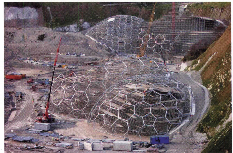
Engineers Anthony Hunt Associates created a 3D model (top) of the foundation “necklace,” which is continuous around the biomes and anchored to bedrock 30 feet below grade. The architect’s early studies (middle) examined how each dome might be subdivided into a feasible structural system. This photograph (bottom), taken in February, shows the first two domes of the warm temperate biome under construction. A model (facing page) shows the biomes as they’ll appear when completed.
