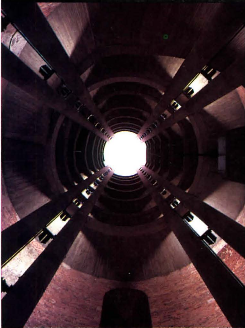
Two concrete slabs in main tower were removed, creating dramatic central shaft above lobby.
