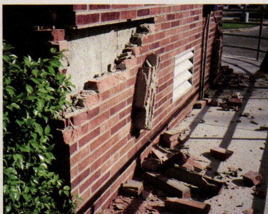
Constructed of unreinforced masonry, First Christian Church in Santa Monica, California, (top) lost its brick facing during 1994 Northridge quake. Sepulveda Veterans Administration Hospital (above), located three miles from quake's epicenter, experienced blowouts at each corner of its brick veneered, reinforced concrete structure.
