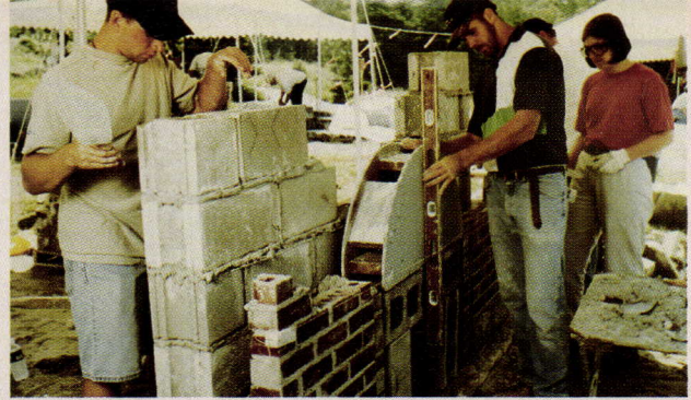
Intern architects and apprentice masons build full-scale wall section of brick veneer over loadbearing CMUs.
