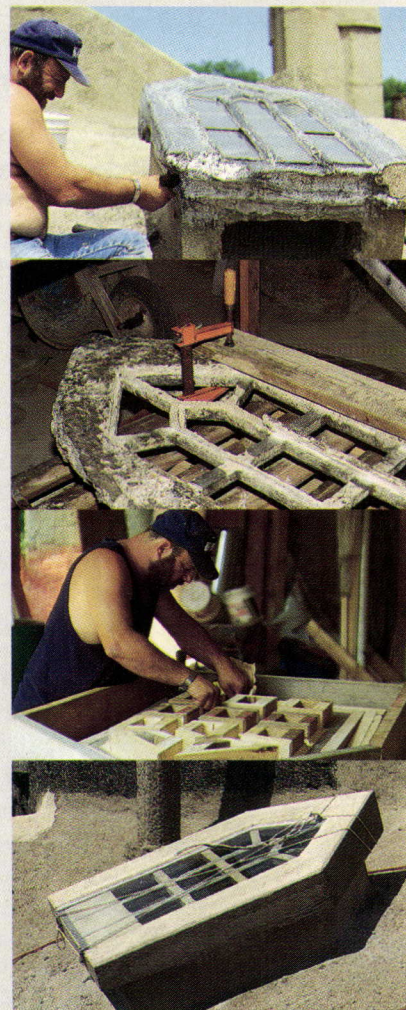
Contractor Denny Griffo removes deteriorated cast-concrete skylight and constructs wood form for casting new concrete window frame.
