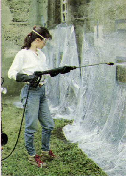
Conservator Catherine Subick removes fungus from concrete with a low-pressure water rinse.
