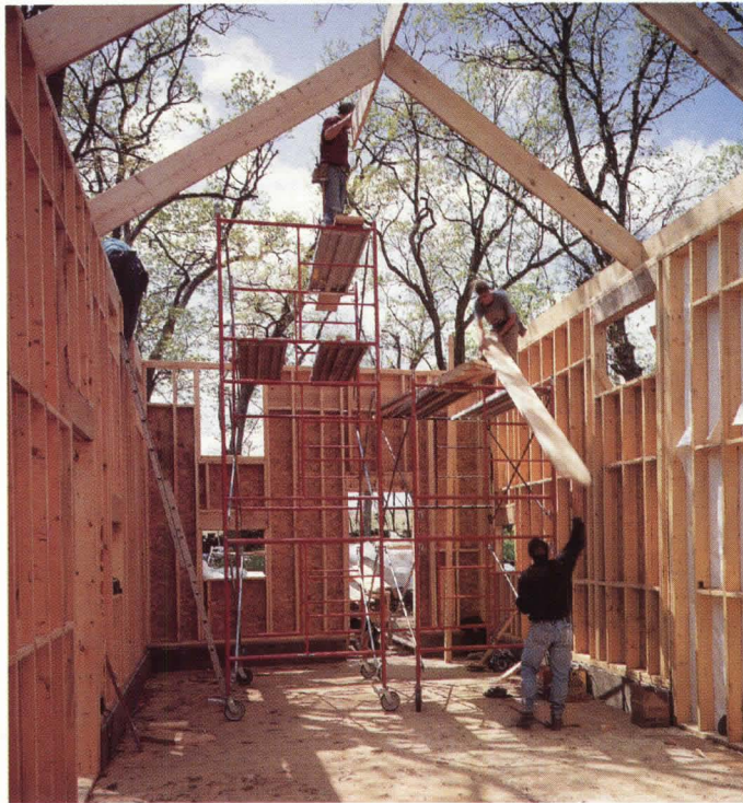
LEFT: KU design/build students install roof framing for artist's studio. BELOW LEFT: Wall sections are erected by students after foundation is poured. BELOW RIGHT: Extruded foundation takes advantage of sloping site. AXONOMETRIC: Students prepared exploded axonometric drawings to explore studio's structural elements.
