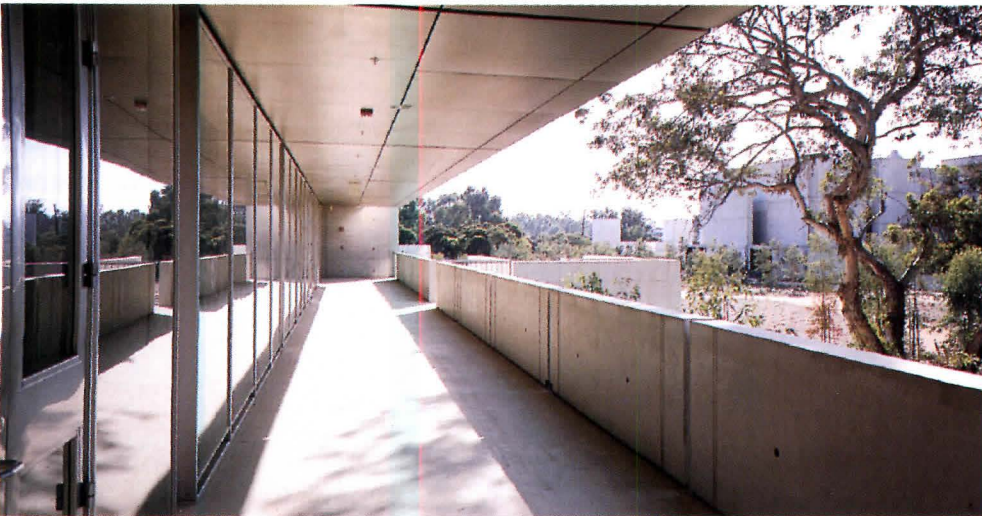
TOP: Upper floor of east facade of south wing is clad in stainless steel screens.
