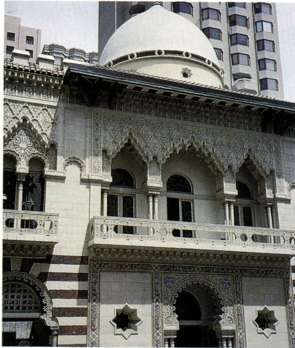
THEATER FACADE: Roof leaks caused terra-cotta damage.
