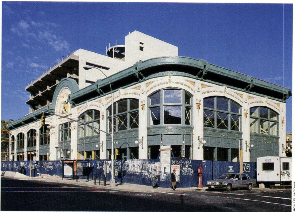
AUDUBON BALLROOM: Polychromed terra-cotta facade restored as part of renovation and addition.
