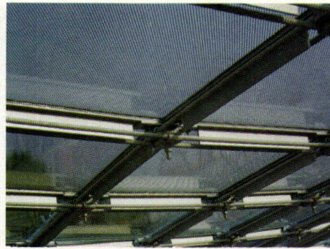
GLASS PANELS: Steel mesh filters sunlight.
