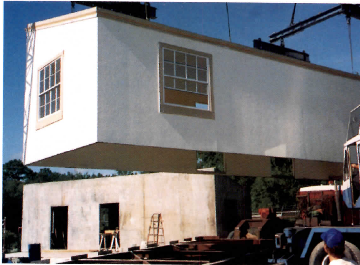
FINISHED MODULE: Two halves of concrete house are joined by precast roof.
