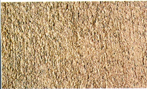
Scraped: A "torn" surface is achieved by scraping the 1/4-inch-thick finish coat after it dries with a trowel held at right angles to the plane of the wall.
