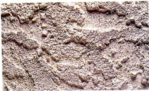
Arizona: A heavy texture coat is applied with a trowel. After surface moisture is absorbed, a second heavy coat is left rough with small areas of texture.
