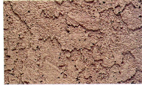
Light Lace: First coat is troweled or dashed to cover base. After the first coat dries, a second coat is applied in random directions and flattened lightly with a trowel.
