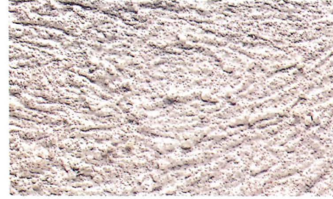
Rock 'n' Roll: A finish plaster coat containing a small pebble aggregate is rolled by a trowel for desired texture. Action of trowel rolls the pebbles to create patterned troughs.
