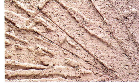
Briar: A first coat is applied by trowel. Texture coat is applied by holding trowel at an angle to the surface. The heel of the trowel serves as a pivot point to produce fanlike ridges.
