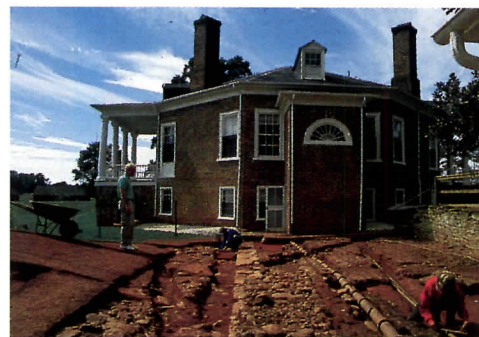
Restoration architects at Poplar Forest (above), Thomas Jefferson's country retreat in Bedford County, Virginia, are writing an historic structures report to determine what elements from the 1806 building are original.
