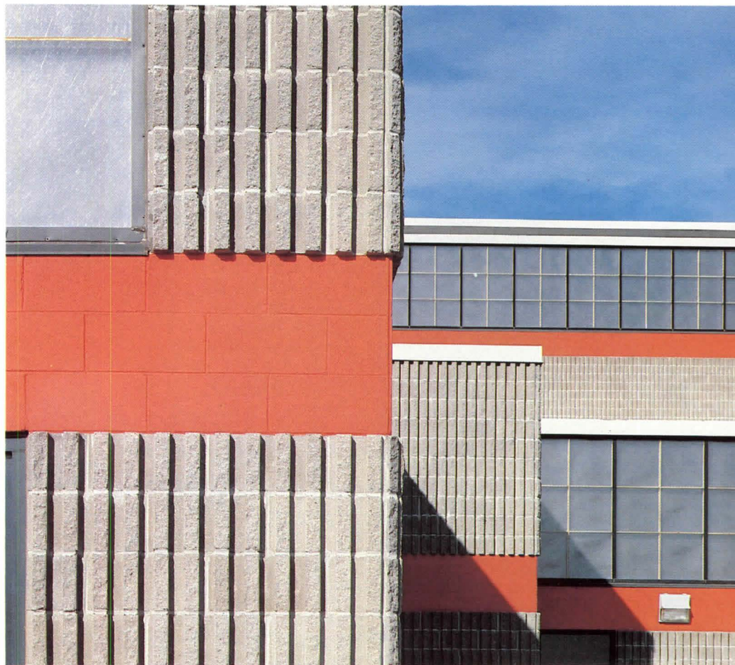
A detail of the concrete masonry exterior walls which utilize split ribbed units and bands of regular concrete masonry. The glazing of the two concrete block Trombe wall sections is seen at the right.
