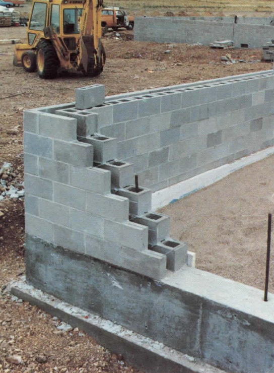
Cavity walls are of 8" concrete block with 4" block veneer. The cores were grouted. Cavities were filled with foamed-in-place insulation.
