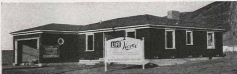
In the Making. Fir-Tex Asphalt Coated Sheathing seals the Life home against sun, wind, rain and dust, and provides an unbroken area of insulation all over the house. Termite proof.
