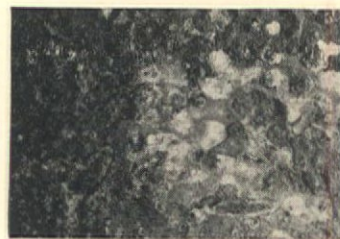
Rust-rotted inside surface of a typical hot water tank after only a few months' service in a region noted for its pure water supply. Engineers cut these old-type tanks open at random . . . found not one that was free from rust or corrosion.
