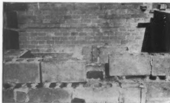
Foundation in foreground is seriously deficient due to improperly filled mortar joints. Filling of holes in block would be an advantage
