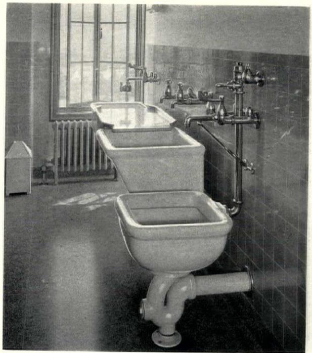
Figure 3. Combination fixtures in nurses' workroom, showing flushing rim hopper, wash tray, scrub-up and work shelf
