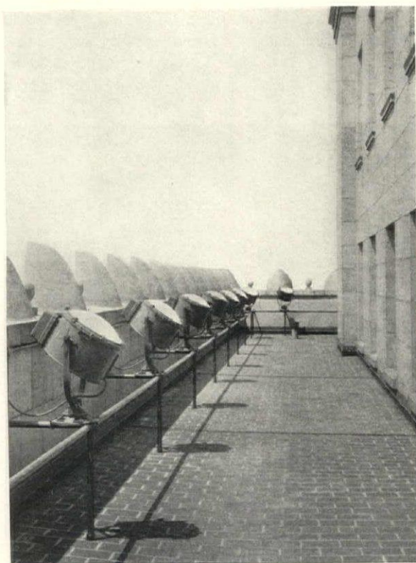
Projectors mounted on the Union Terminal Building
