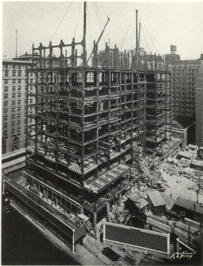
The Palmolive Building, showing steel frame with wind bracing and pan system of structural floor construction. Holabird & Root, Architects
