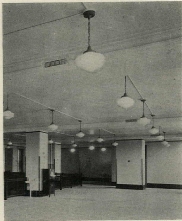
Office Lighting Showing Development of Circuits from Central Outlets by Using Metal Moulding Conduit
