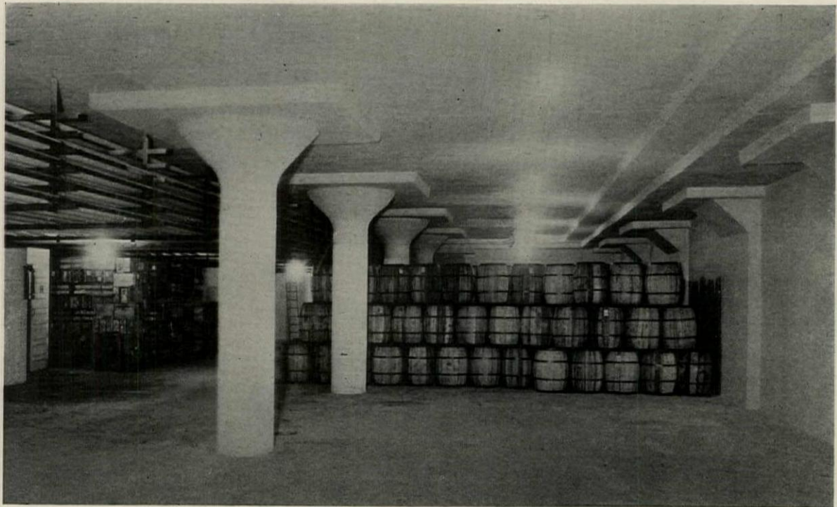
Interior of Quaker City Cold Storage Warehouse Showing Construction The Ballinger Company, Architects and Engineers
