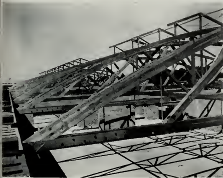
◀ Corner detail of the glued laminated bowstring truss. Note simplicity of detail of these trusses used in another structure. Top and bottom chords are glued, made up from 1½ inch material.
