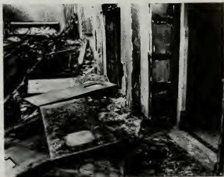
These swinging doors in the Lynn High School were a major factor in saving the balance of the school when the auditorium section burned with a loss estimated at $250,000.
