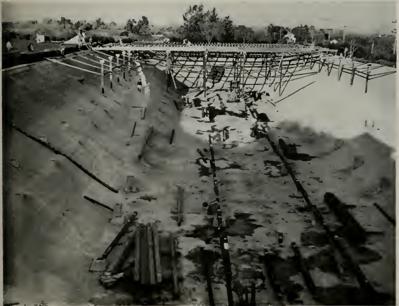
CAMBRIA RESERVOIR, California Water Service Company of San Jose, California, showing a type of work being featured by the Stolte Company along with roads, pipe lines, and other heavy construction.
