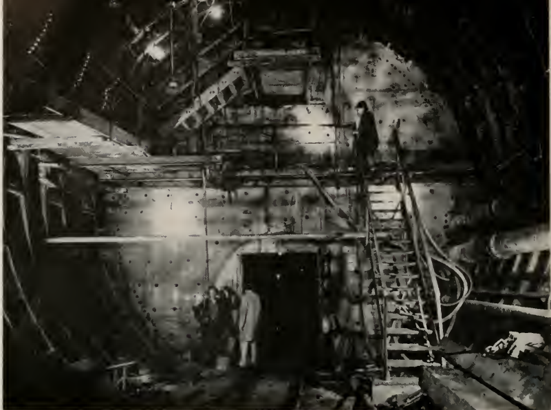
WORK advances behind a heavy iron shield, moving forward 32 inches at a time to permit the next ring to be anchored.
