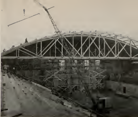
CRANE with jig boom lifts purlins into place and also lifts decking for huge roof area.
