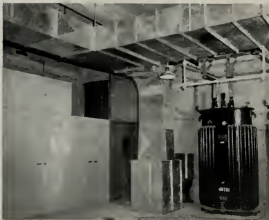
OVERHEAD sheet metal air ducts feed cold air from the blowers.
