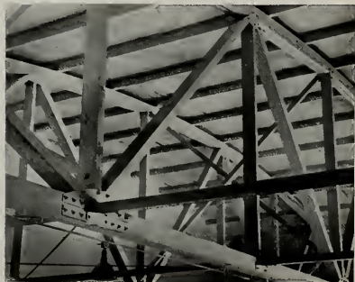
CLOSE-UP view of roof and truss members shows strength of Monochord design. Complete rigidity is had and obstructing pillars are eliminated.
