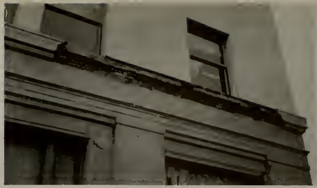
Looking west at Benjamin Franklin Life Building, Santa Barbara, California. Fallen facing from east side of north corner.
