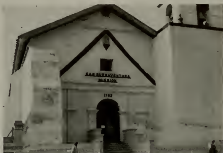
Looking north. Mission at Ventura, California. Brick building with concrete stucco veneer. New cracks in veneer but many cracks are old ones.
