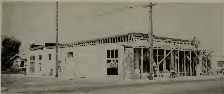
Looking east at Drug Store building, Carpinteria, California. 1-story concrete block building. Front and side walls fell into street.
