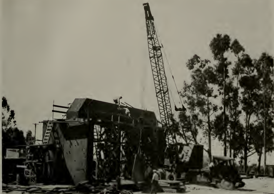
MORE THAN 4900 TONS OF STEEL, ALL ARC WELDED, USED IN CONSTRUCTION OF THIS MONSTROUS STRUCTURE AT UNIVERSITY OF CALIFORNIA, BERKELEY
