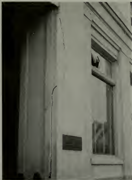
Looking west at Benjamin Franklin Life Building, Santa Barbara, California. South side of entrance.
