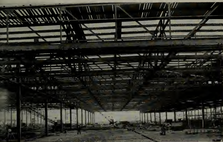
Steel frame of one of the huge assembly buildings under construction for the Douglas Aircraft Company, Inc., at North Long Beach, California. Outside bays are 30 feet and are increased to 60 feet on the inside to provide clear assembly areas.
