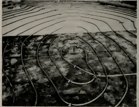
GAS-FIRED PANEL HEATING EQUIPMENT INSTALLED IN FLOOR
