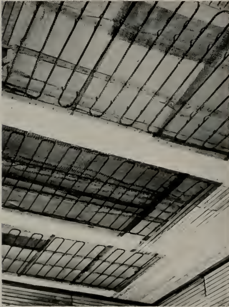
GAS-FIRED PANEL HEATING EQUIPMENT INSTALLED IN CEILING
