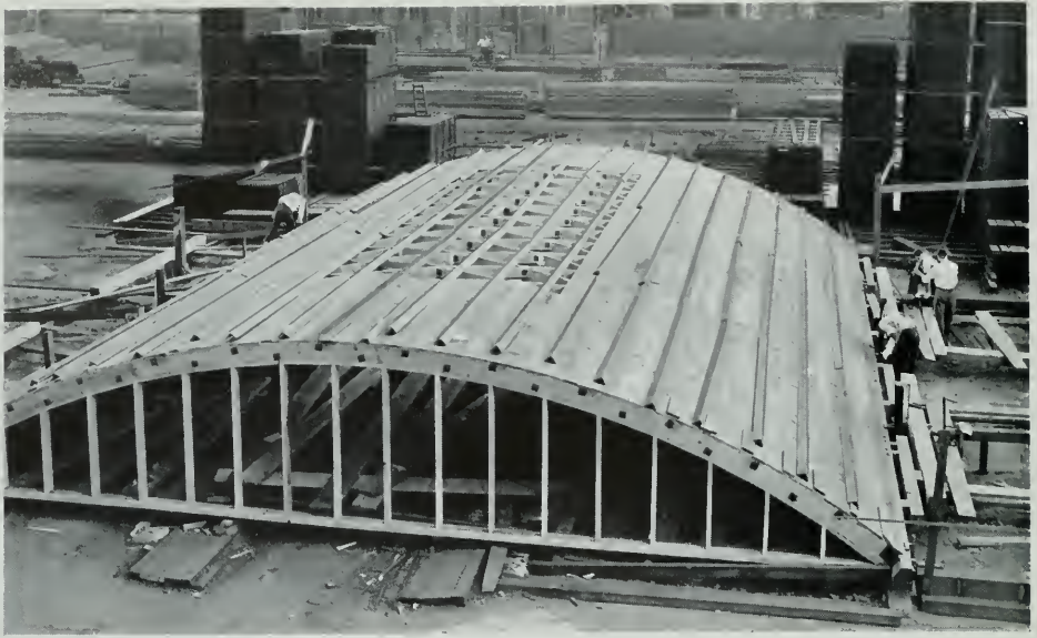
LAMELLA TEST ROOF DURING FINAL EXPERIMENT. SHEATHING REMOVED ON CENTER OF ROOF. END DIAPHRAGM SHEATHING REMOVED LEAVING ENDS UNSUPPORTED. STEEL ANGLES APPROXIMATE WEIGHT OF ROOFING. IN THIS TEST A LATERAL LOAD OF 390 POUNDS PER LINEAL FOOT OF SILL WAS APPLIED ON THE WEST SILL ONLY.
