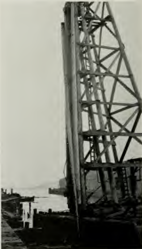
Photograph shows removal of piles at Pier 19, San Francisco waterfront, October 26, 1937, to make room for new pier. Note excellent condition of piles after service of 23 years. The piles were originally treated with West Coast Wood Preserving Company's creosote, represented in San Francisco by J. H. Baxter Company.
