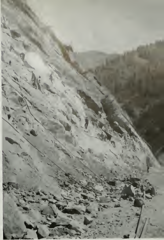
"IN THE MAKING"—BLASTING A SECTION OF A NORTHER CALIFORNIA HIGHWAY, FEATHER RIVER, PLUMAS COUNTY
