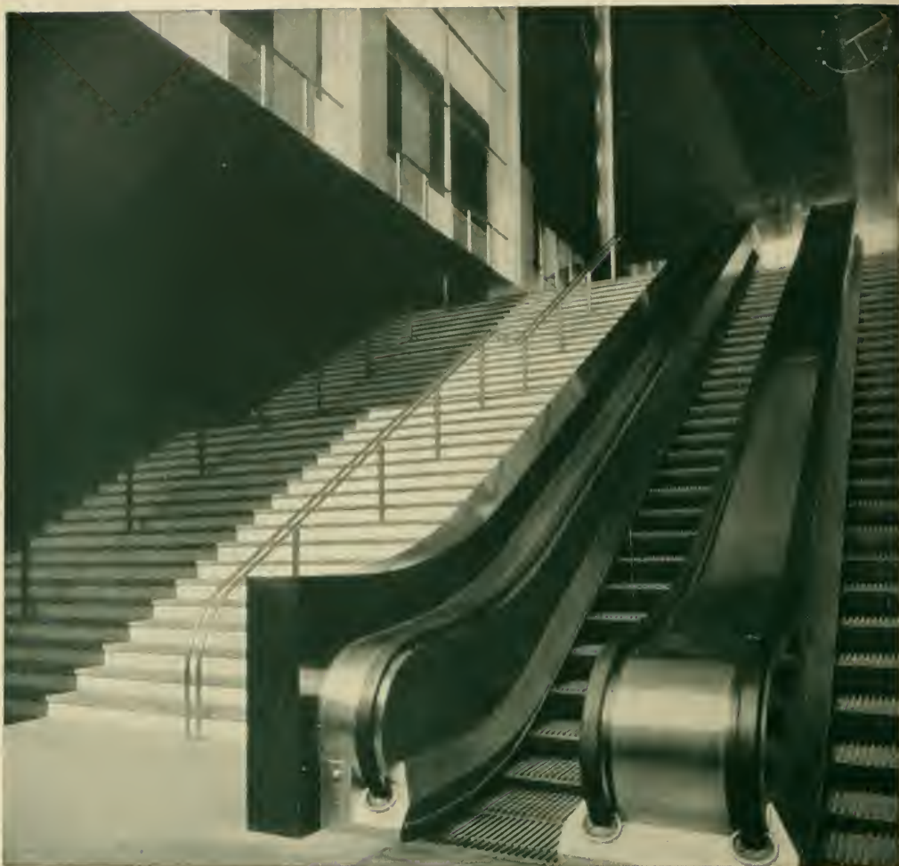
Photograph of escalators in the new building of The Philadelphia Saving Fund Society
