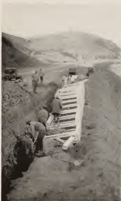
Metal crib wall, 114 feet long, installed by the California Division of Highways on Bayshore Highway, two miles south of the San Francisco-San Mateo County line.
