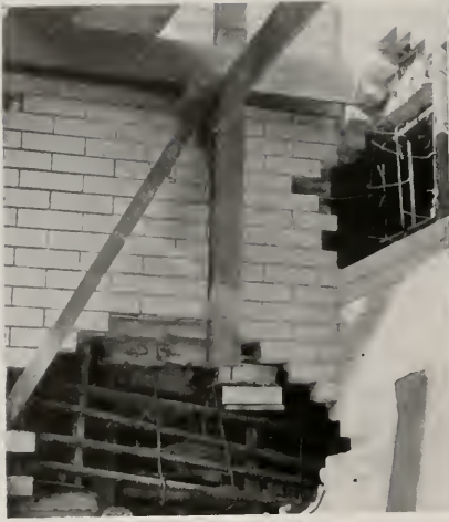
Above—View of preparation of walls and steel assembly at a wall corner.
