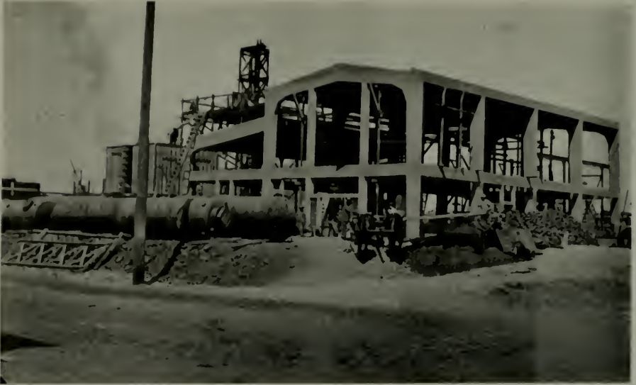
FIG. 6.—CONCRETE FRAME, SULPHUR DIOXIDE BUILDING, AVON, CALIFORNIA Engineering Department, Associated Oil Company
