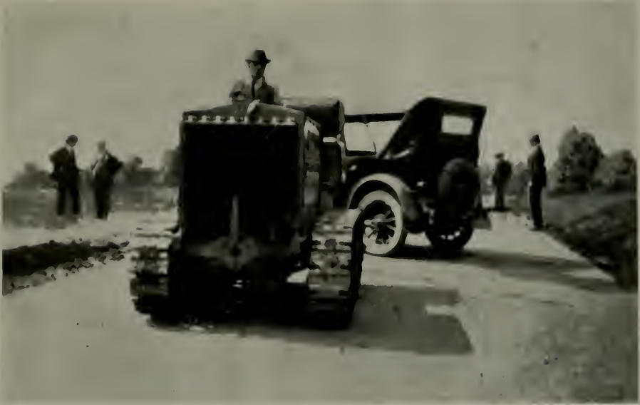
This pavement, made of Atlas Lumnite cement, carried heavy traffic the day after construction. Illustration shows fifteen ton oil distributor and ten ton tractor being driven over pavement twenty-four hours after being laid.
