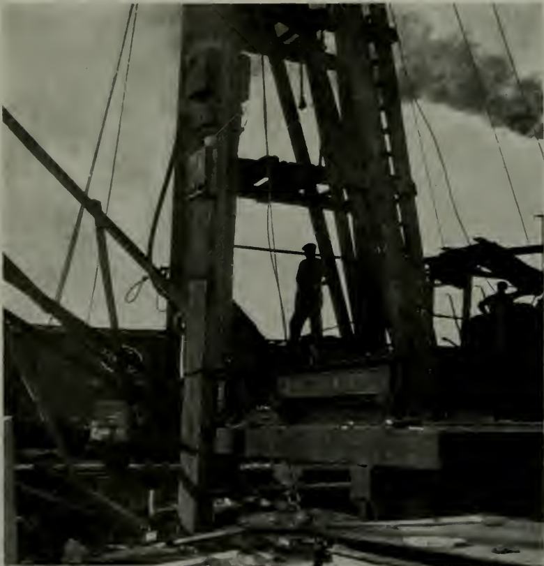
Driving an eighteen-inch octagonal pile 25 feet long and made of Lumnite cement, twenty-six hours after casting. McLain Contracting Company, Baltimore.
