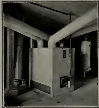
A No. 80 Babcock Furnace installed in the home of Dr. C. A. Abramopoulos, 886 Twenty-fifth avenue, San Francisco.
