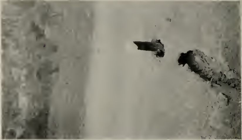
WARNING SIGNAL, PLACED IN HOLE IN THE ROAD CAUSED BY BURNING OUT OF WOODEN CULVERT ON WILDCAT CANYON ROAD,
