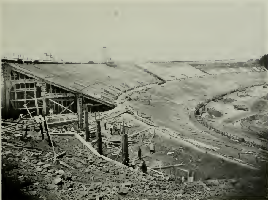
CALIFORNIA MEMORIAL STADIUM, BERKELEY Showing method of suspended slab and beam construction
