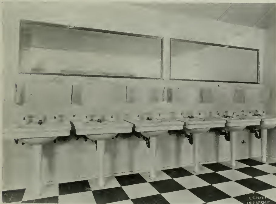
ONE THOUSAND AND SEVENTY-EIGHT OF THESE LAVATORIES IN THE NEW BILTMORE HOTEL, LOS ANGELES, FURNISHED BY PACIFIC SANITARY MANUFACTURING CO.
