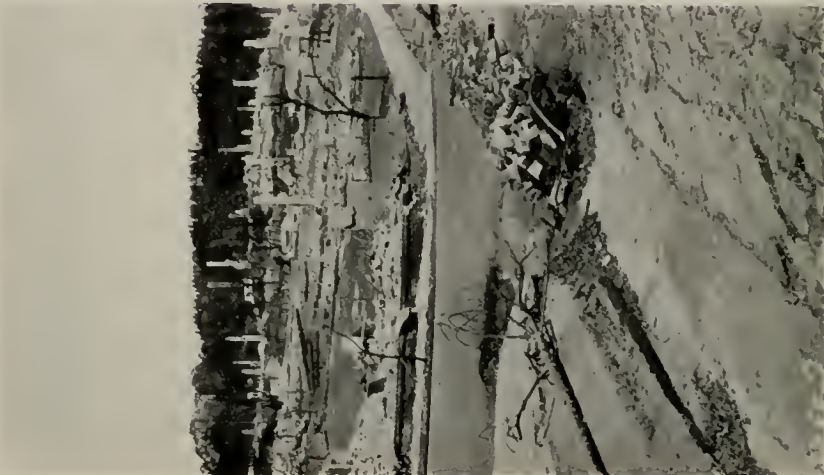
BURNED OUT WOODEN CULVERT IN THE AREA DEVASTATED BY FIRE, BERKELEY, SEPTEMBER, 1923.
