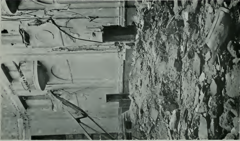
Showing truss T-12 against the 18th Street wall. Note terra cotta above ceiling line upon which truss rested.
