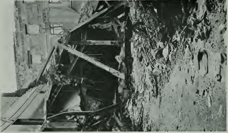
The much discussed column C-2, showing that part above the joint whose upper end rests on the floor. The greatest strain fell upon this column.
