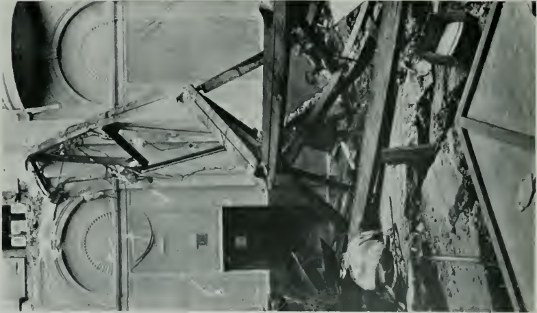
Truss T-12 up against the 18th St. wall. Note ventilating fan at left, which was carried down by collapse of the concrete roof.
