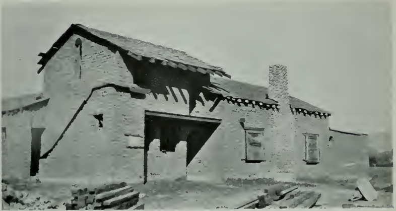
ADOBE HOUSE FOR MR. H. R. JOHNSON, BRENTWOOD PARK, UNDER CONSTRUCTION John Byers, Designer and Builder
