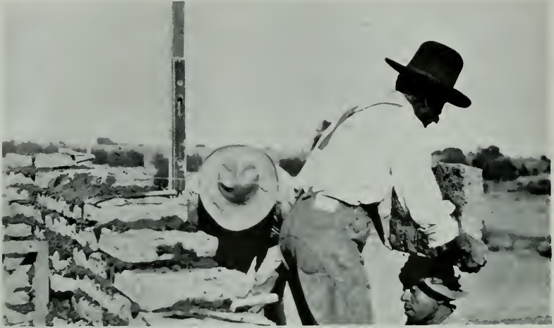
CARRYING AND SETTING ADOBES. HOUSE OF MR. H. R. JOHNSON John Byers, Designer and Builder
