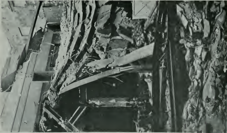
Intersection of Columbia Road wall and south wall. On the left, column C-2 and that part above the joint broken off. Here is an excellent presentation of what came down on the heads of the spectators. The concrete roof is only three inches thick.
