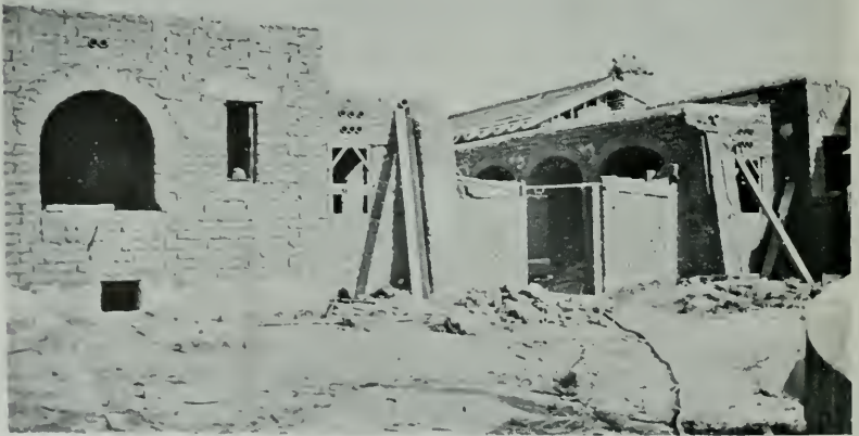
ADOBE HOUSE FOR MR. ARTHUR ROSSON, BEVERLY HILLS, CAL., UNDER CONSTRUCTION John Byers, Designer and Builder
