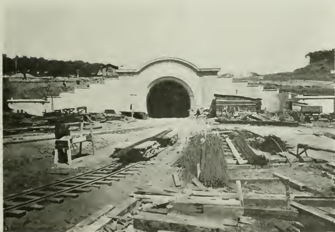
WEST PORTAL, TWIN PEAKS TUNNEL, SAN FRANCISCO M. M. O'Shaughnessy, City Engineer
