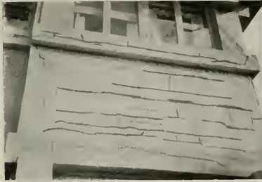
FIG. 5—Section of cement-plastered residence. Note defects due to absorption of water.
