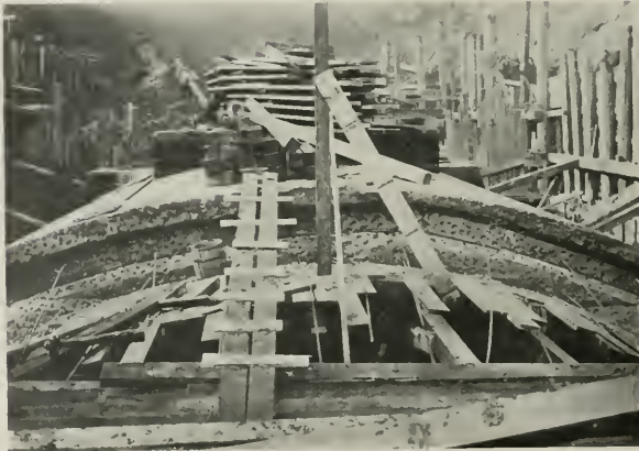
CONCRETE ARCH IN TUNNEL SECTION CONSTRUCTED IN OPEN CUT, SHOWING KEY AND ROUGHED SURFACE FORMING CONSTRUCTION.
