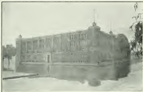
San Francisco Armory Now Under Construction California State Engineering Dept., Jno. W. Wolcott, State Architect
