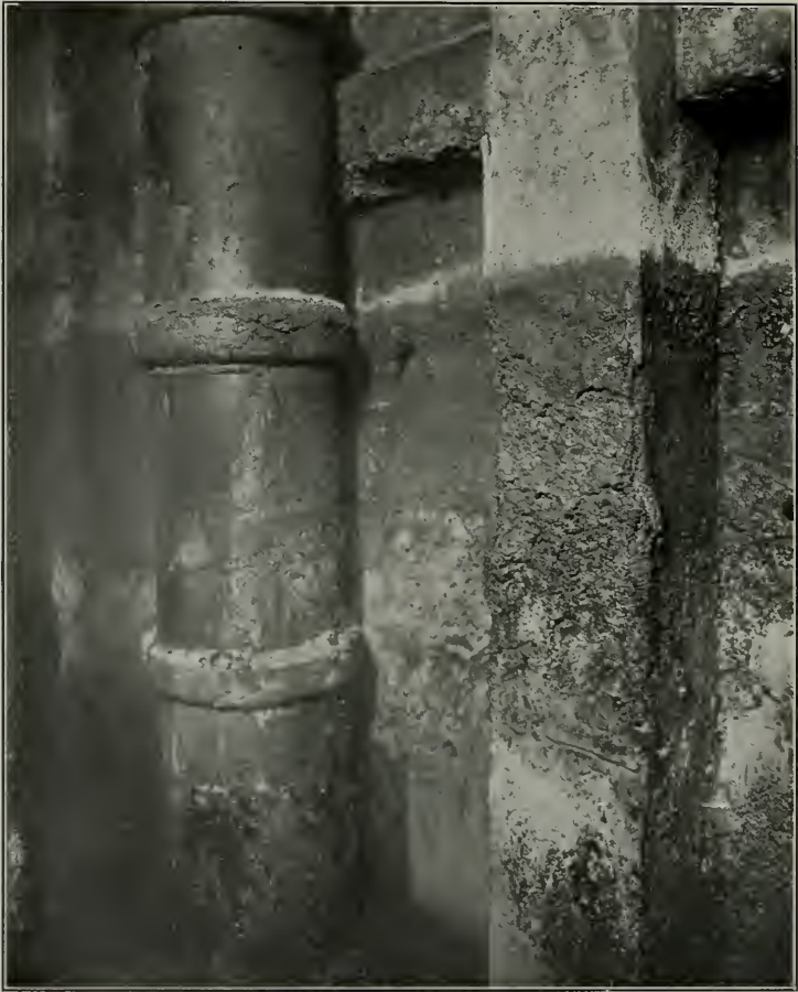
Septic tank at California State University Farm, built about 1908; photo taken October, 1911, showing concrete in effluent chamber disintegrated by domestic sewage, while the vitrified clay pipe remained in perfect condition. The floor of the effluent chamber of this septic tank is some seventeen feet below the surface of the ground.
