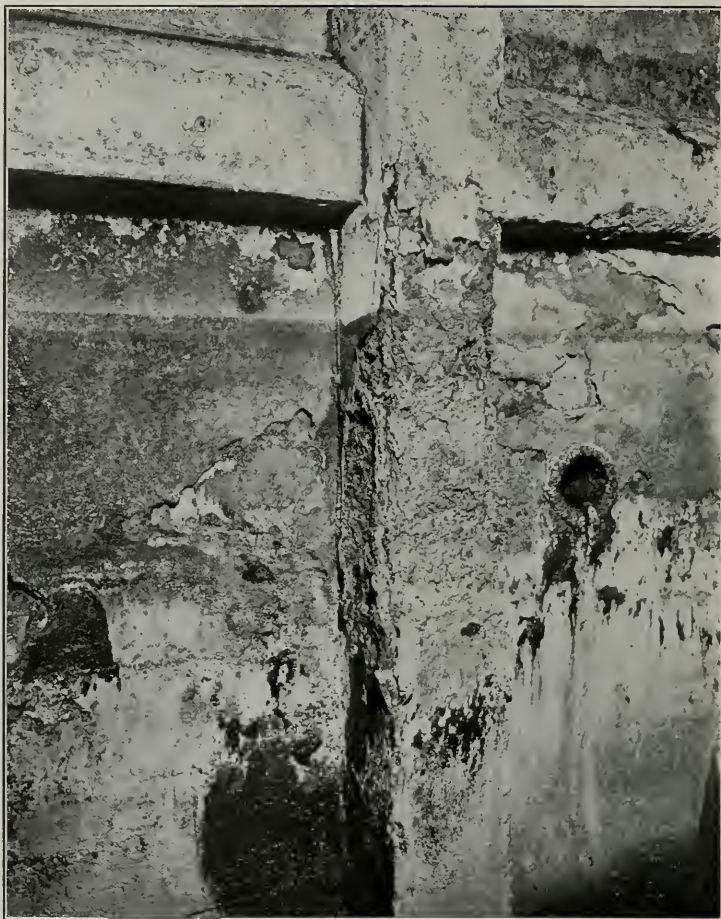
Septic tank at California State University Farm; built about 1908; photo taken October, 1911, showing concrete in effluent chamber disintegrated by domestic sewage.
