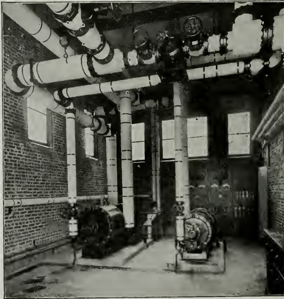
Steam Turbines and Piping in the School Power House
