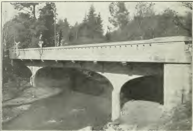
Fig. 4—Reinforced Concrete Girder Bridge, City of Ross, Marin County, California John B. Leonard, Engineer
